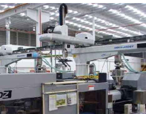
INSTALLED ON SUMITOMO MACHINE
